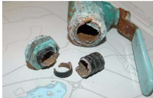
An example of corroded assembly.
